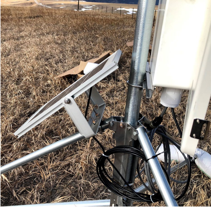
Figure 8. Fully assembled solar panel and enclosure
